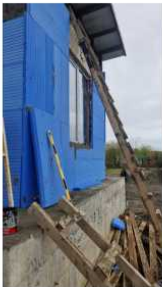
Unsafe handmade ladder
