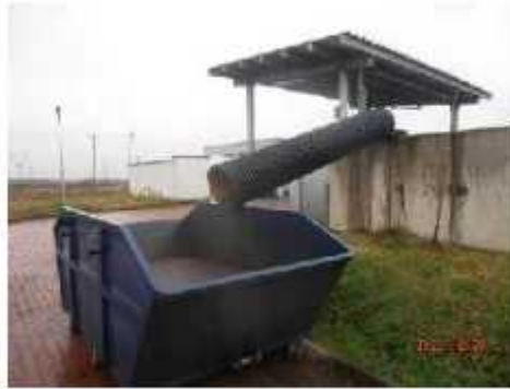
Dried sludge at emergency storage hall
