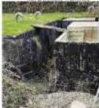
BIGI Reservoir - Not protected Trenches
