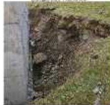
Averoni Reservoir - Dangerous Trenches
