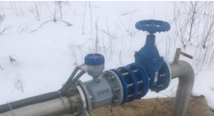
PHOTO No1 – WELLFIELD BOREHALL N1
