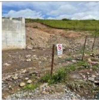
Construction sites be properly fenced from all sides with lockable gate
