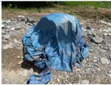
Construction materials be stored properly
