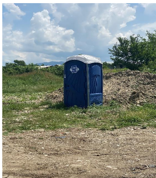
Bio toilet provided at the construction site
