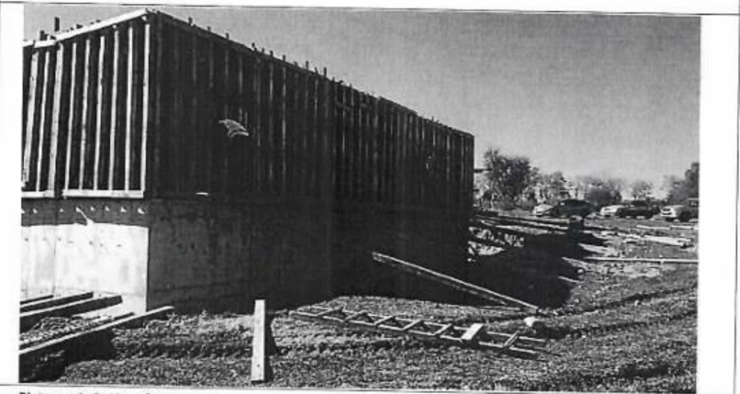
Pictures 1. 2. Unsafe activities
