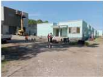
Area around the cherry picker without warning tape
