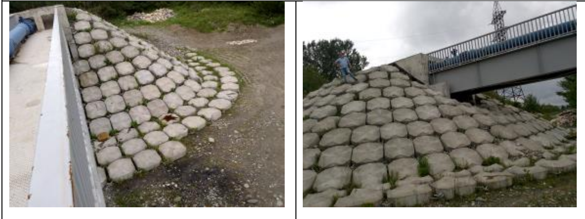
Figure 6 and 7: The restored slopes in the area where the Rioni River is intersected with the water supply pipeline
