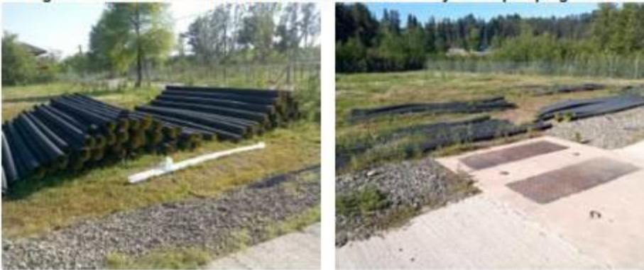
Figure 16 and 17: The construction waste on the territory of the pumping station
