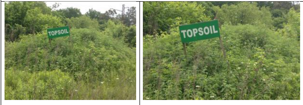
Figures 8 and 9: Topsoil left uncontrolled in the area of temporary disposal (Mukhrani Pumping Station)
