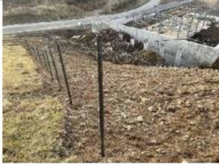
Construction sites should be properly fenced
