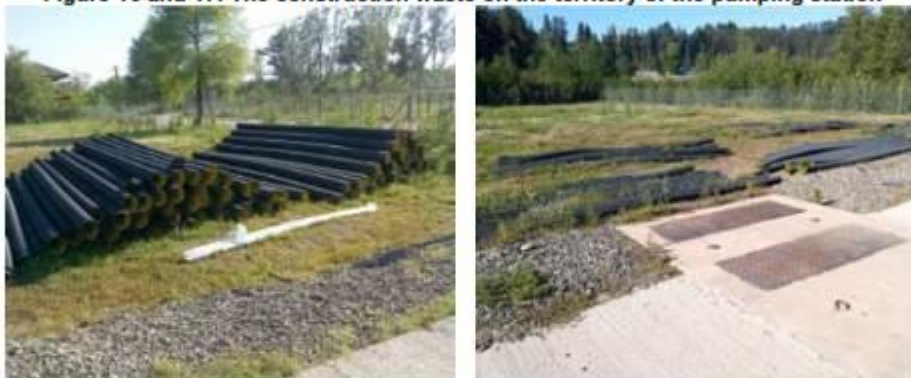
Figure 16 and 17: The construction waste on the territory of the pumping station
