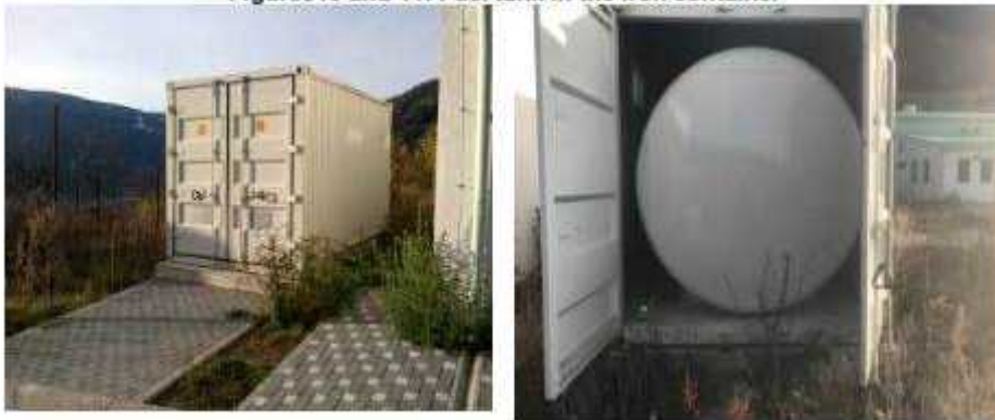
Figures 10 and 11: Fuel tank in the iron container
