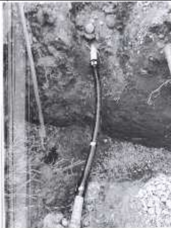
Figure 6: Damaged underground infrastructure and the same section after rehabilitation – Agmashenebeli Str.
