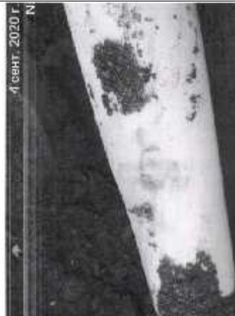
Figure 2: Damaged underground infrastructure and the same section after rehabilitation – vil. Culukuze
