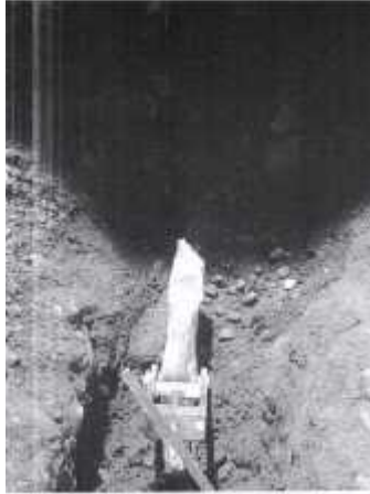
Figure 1: Damaged underground infrastructure and the same section after rehabilitation – Rustaveli Str.
