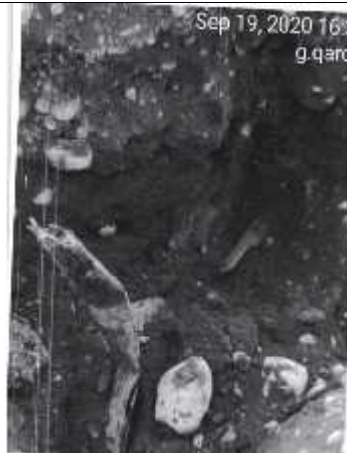
Figure 3: Damaged underground infrastructure and the same section after rehabilitation – 8 March Str.
