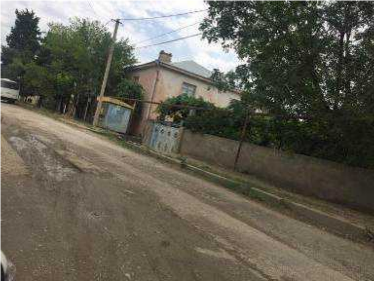
CHI-01 – Improper reinstatement of road after laying of sewerage line (Photo-01)
