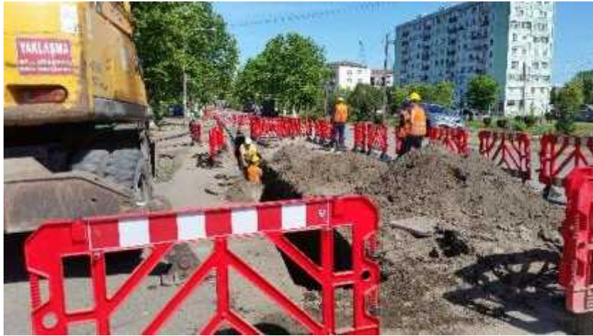
Photos POT-01, Construction of Sewerage Systeem in Poti (Photo No22, Photo No23, Photo No24, Photo No25)
