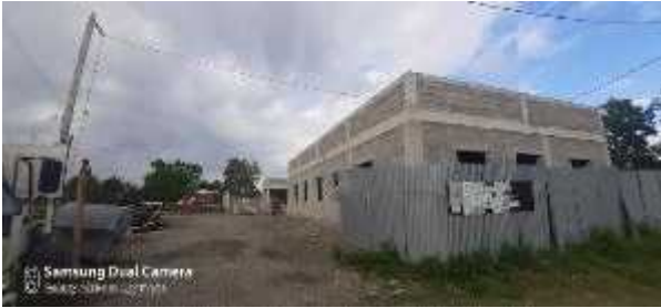
Abasha - UWSCG's Service Center area, construction getting towards the end; front view, Photo-06
