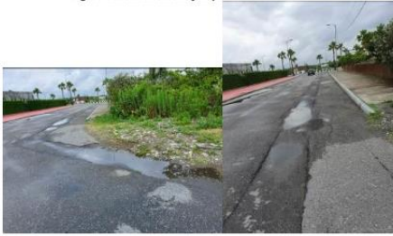
Figure 10. Unsatisfactory asphalt restoration works
