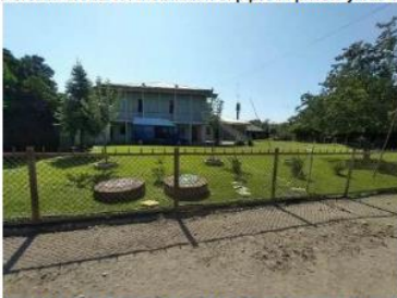
Figure 4. Restoration Works for installation of pipes in private yards of the families
