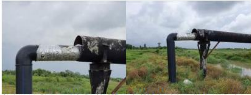
Arraignment of pressured pipeline ( d= 355 \text{ mm} , l= 1813\text{m} ) and connection to existing l= 2400\text{m} same pipe; Arraignment ramp connection on the main channel with a steel casing pipe ( d=630\text{mm} l 9\text{mm} , l= 21\text{m} )
