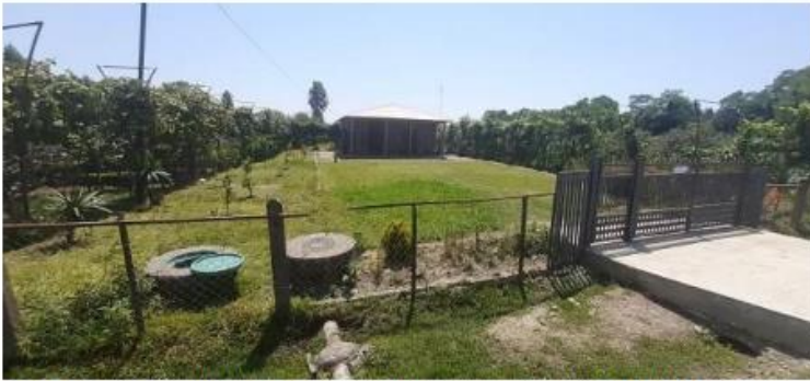
Connection of residential houses in Anaklia resort to main sewer line. Corrugated d=150mm sewer pipe. Rustaveli street.
