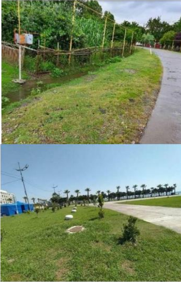
Figure 3. Restoration Works for installation of pipes in urban area of Anaklia and Ganmukhuri
