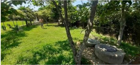
Connection of residential houses in Anaklia resort to main sewer line. Corrugated d=150\text{mm} sewer pipe. Pirosmani street.
