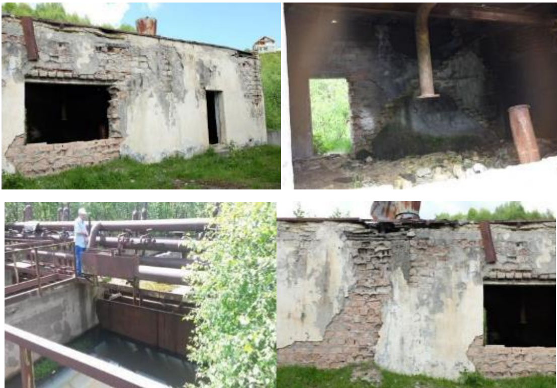
Figure 1: Photos of Ruined Old Waste Water Treatment Plant in Gudauri
