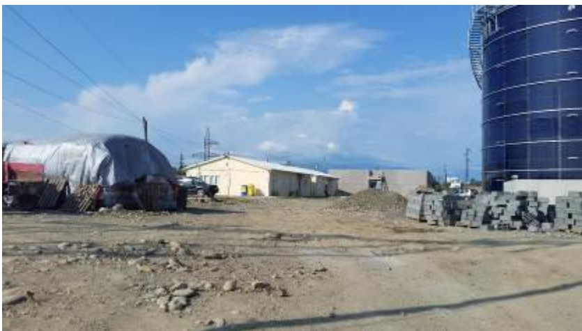
Photo 1: Electric Cables at the Construction Site
