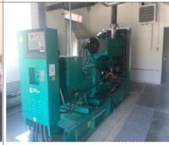
Figure 6: The generator is placed on the secondary protective tank
