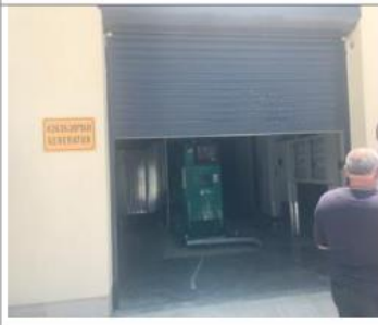
Figure 5: The generator is placed in a covered area
