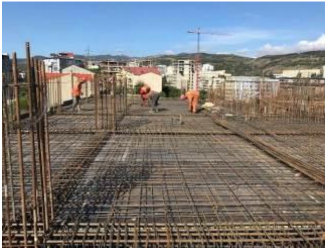
Photos: Construction of the Water Supply Network in Ureki (Ure-01) Laituri Reservoir #2
