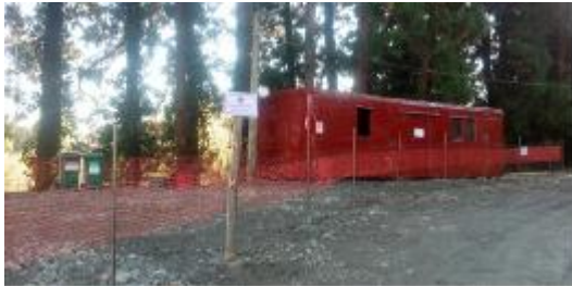
Ure-01 – Pumping Station
