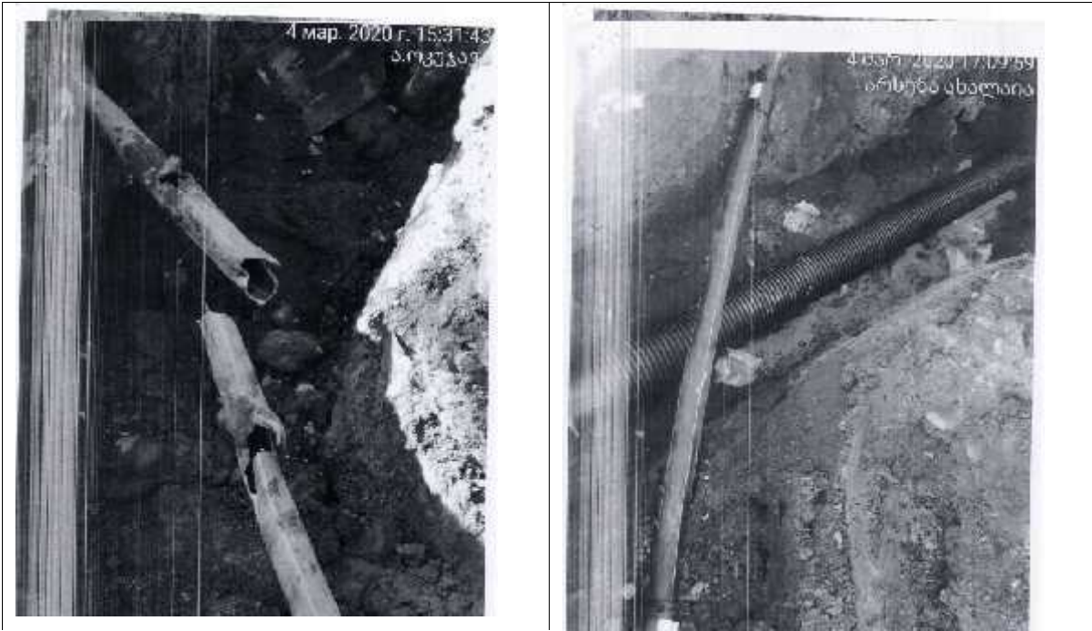
Figure 4: Damaged underground infrastructure and the same section after rehabilitation – Esebua Str.
